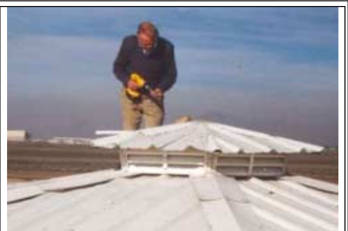
Dennis Cullum repairs the cupola that was blown off the hangar 3 roof.
